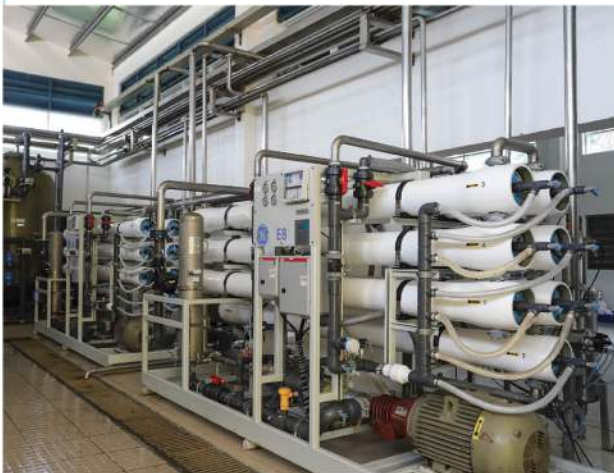
Beer brewing water treatment area
