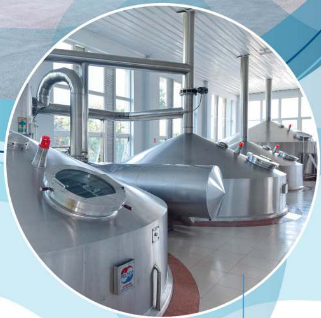
Hot steam recovery system for energy saving system
